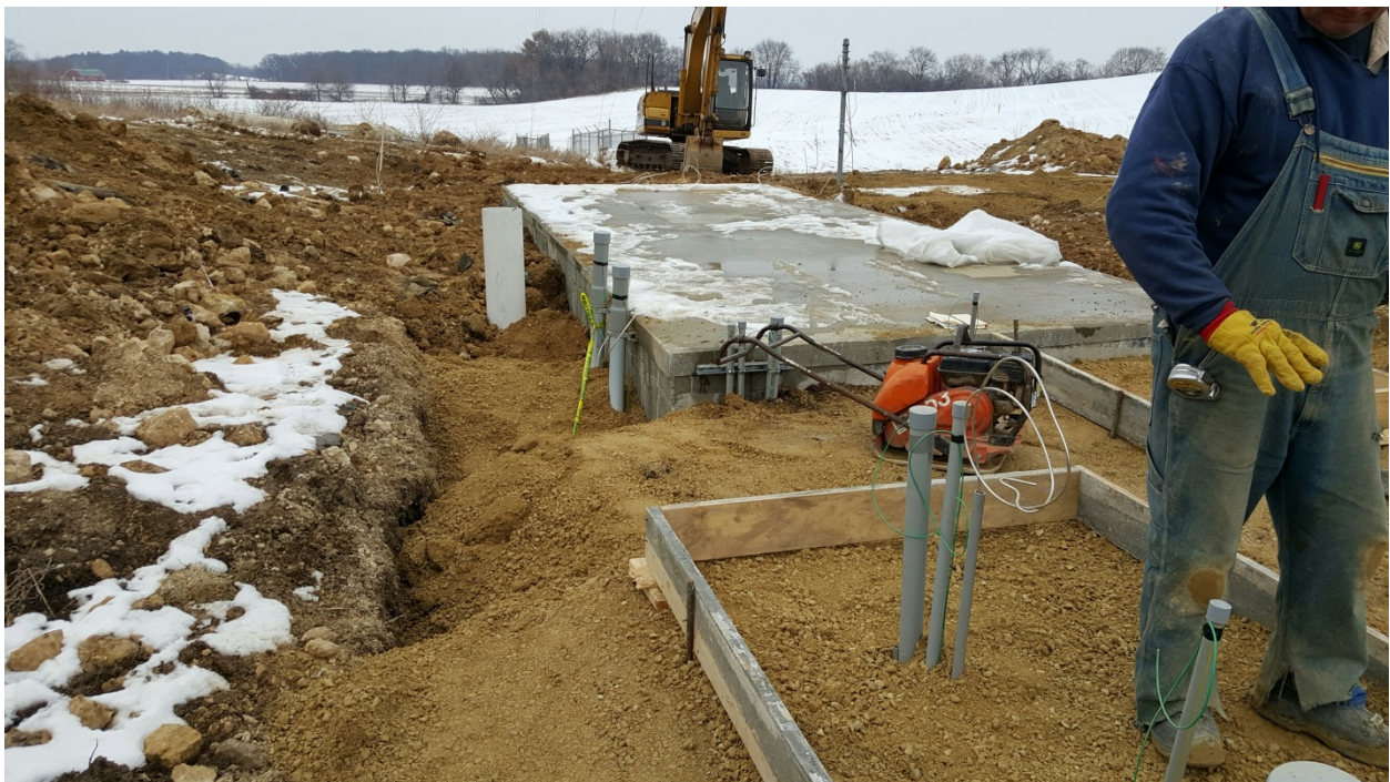
Rockdale tower site. Concrete pad for the equipment shelter is seen. The shelter will be delivered in the coming weeks. The shelter is trucked to the location whole, and (not so) simply set and secured onto the concrete pad you see here.
